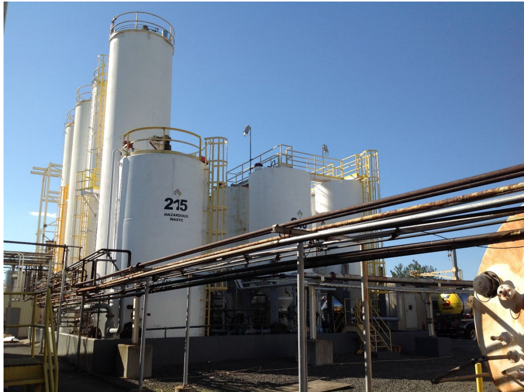
Photo 26 – Tank Farm 2 (Southeast Side)
